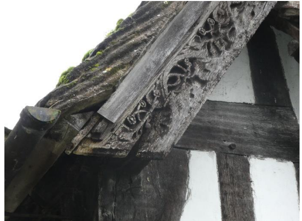
Decaying original bargeboard to front gable.
