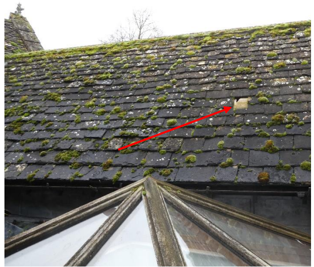
Hole in roof over Tourist Information Centre.
