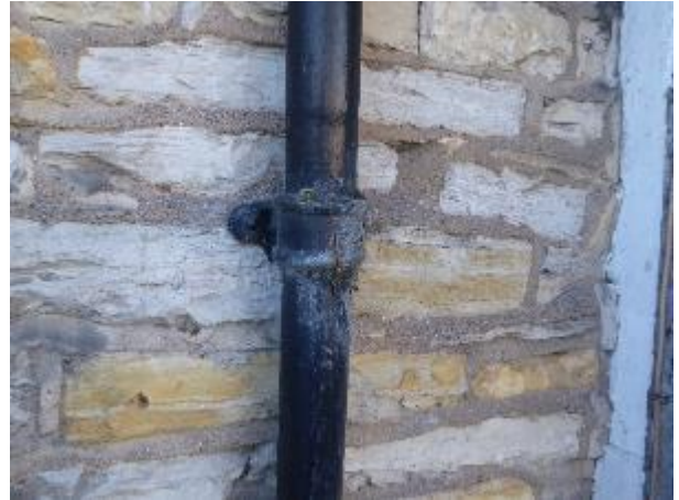
Fractured rainwater pipe - North side
