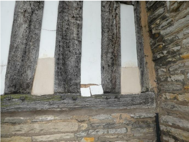
Repaired and failing panels.
