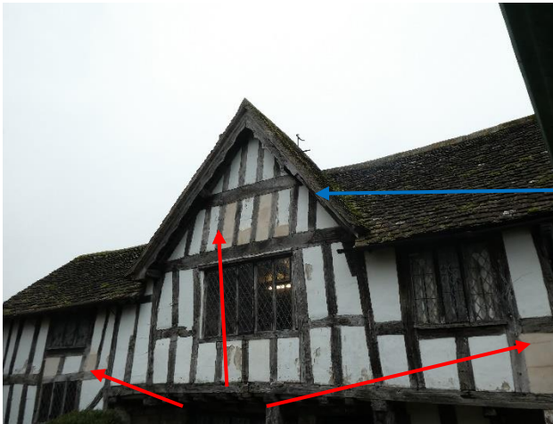
Recently patched panels to south wall following falls.
