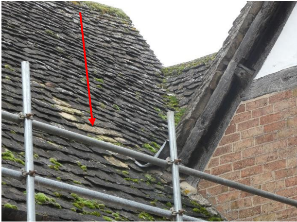
Recent slate repairs following fall onto Kitchen Lean-to roof.
