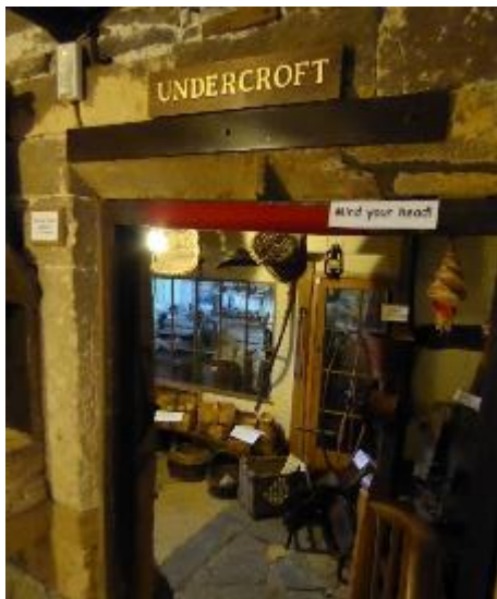
Crude strapping to Undercroft door lintel
