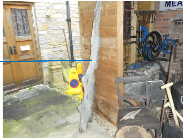
Fallen decayed original bargeboard- former location arrowed.
