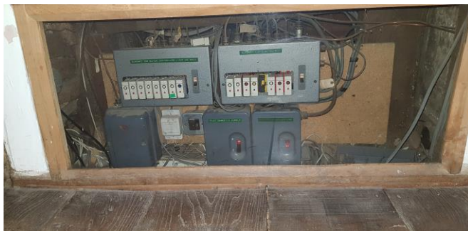
Contactor controlled DB on the left.
