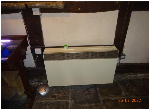
Typical Storage Heater
